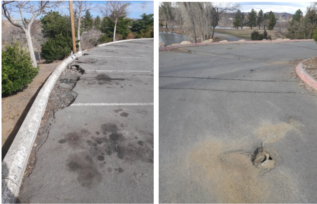
Parking lot damage from rodents
